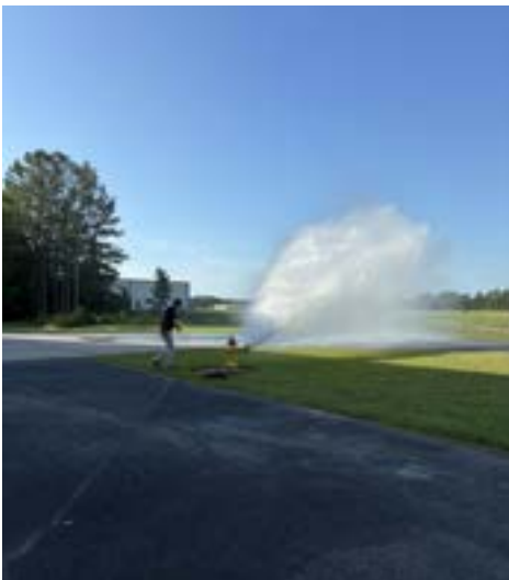
This is "our" hydrant. The other belongs to the city."
